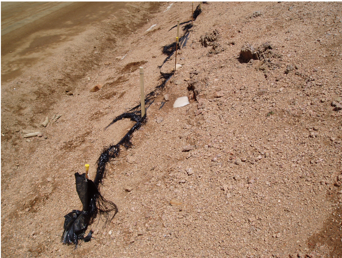
Figure 3. Condition of lower silt fence at site 123CS in spring 2004.
