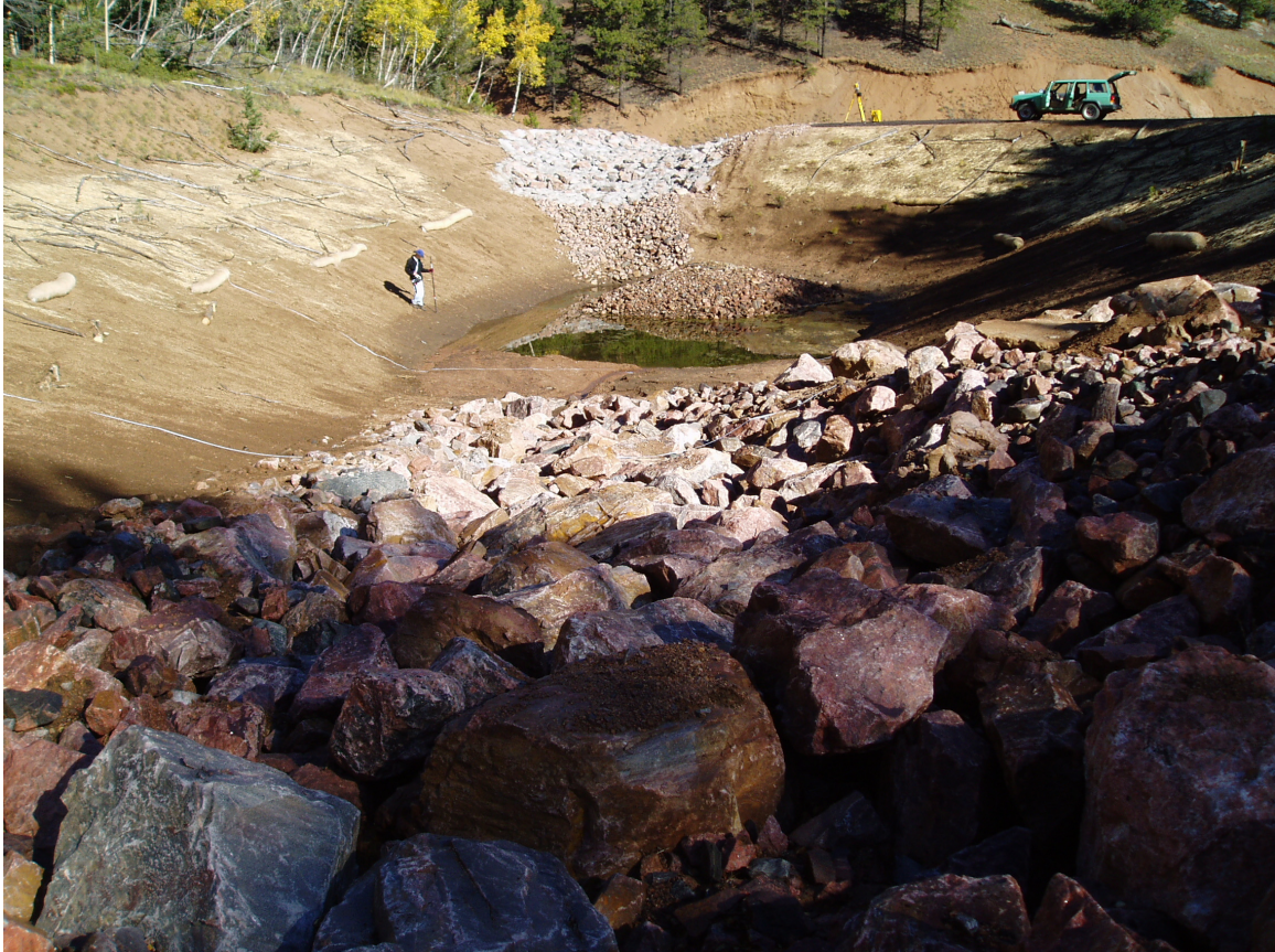
Figure #9. View of sediment pond 199RW from XSA in conveyance channel looking north. Note large rock in channel (forefront), rip-rap from grouted spillway down to the pond, erosion control measures within the basin such as excelsior logs, erosion control fabric, and woody debris.
