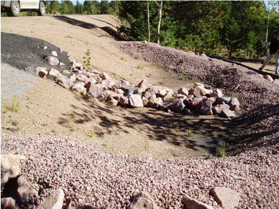
Figure 7. Example of rip-rap velocity dissipator in rock weir 161RW.
